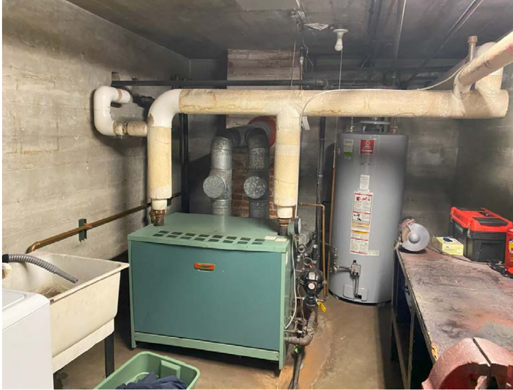
Photo 27: Utility room in basement.
